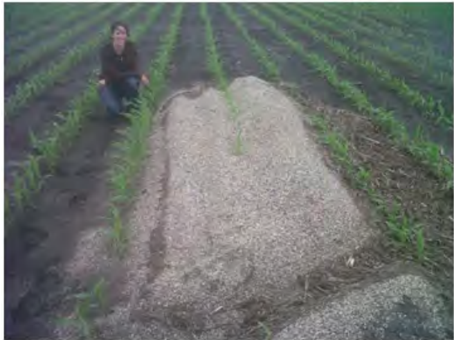
Underground Tile Intakes
