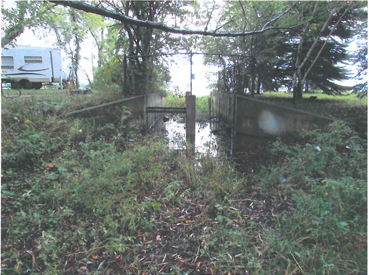
Figure 4. Photo of existing water control structure/fish trap on the outlet of Garlock Slough. Carp barrier is no longer functioning and the outlet channel is filled with sediment.
